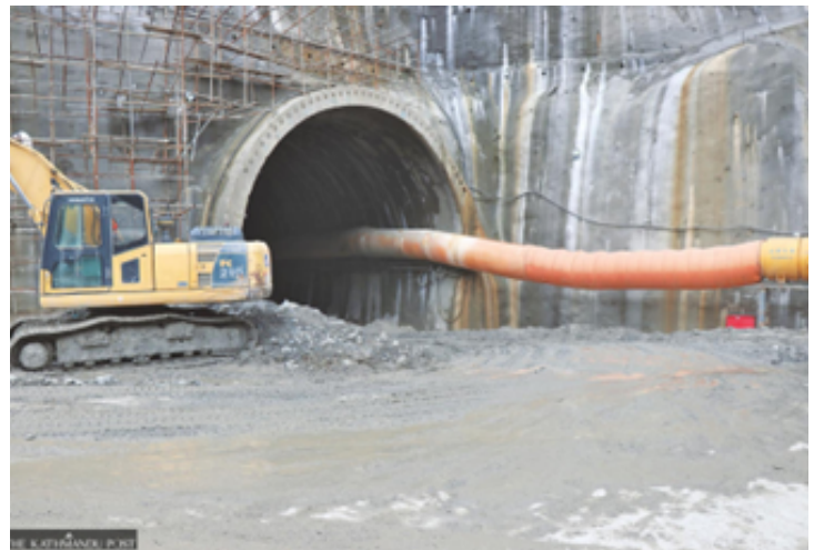
Fig. Tunnel in Siddhababa (focused on bypassing the 4 km hazardous section) (Source: The Kathmandu Post, September 26, 2024)
